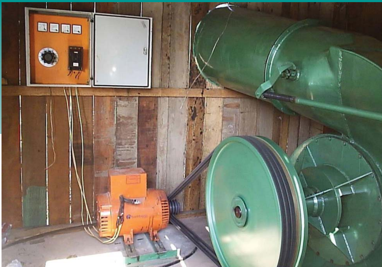
Micro-hydropower turbine and generator, part of a pilot project to install a renewable-energy "mini-grid" for the remote village of Cachoeira do Aruã in Brazil, 145 km from Santarém up a tributary of the Amazon. Photo credit: Indalma Industria/Nazareno Natalino/USAID.
