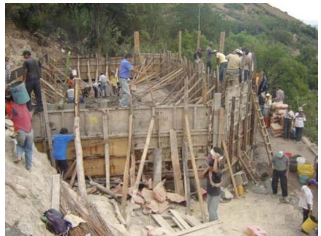
Farmers, villagers, and local officials build a reservoir to supply water to farms in Santa Rosa de Ocana, in Ayacucho, Peru. Photo credit: USAID.
