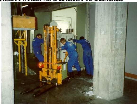
Picture 54: Phase out of an intact PCB transformer
