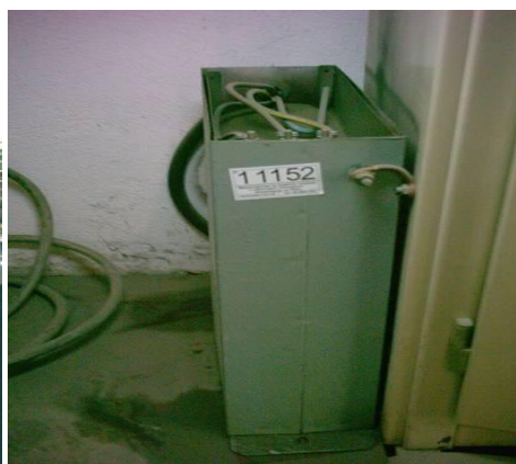
Picture 56: Inventoried and labelled capacitor
