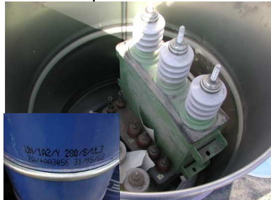
Picture 68: PCB capacitors in steel drum
