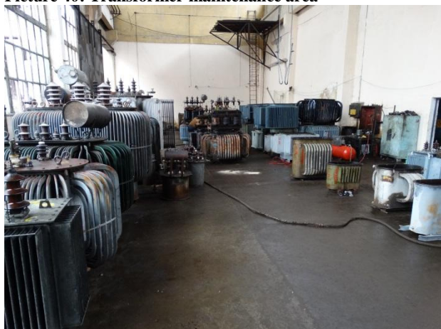
Picture 40: Transformer maintenance area
