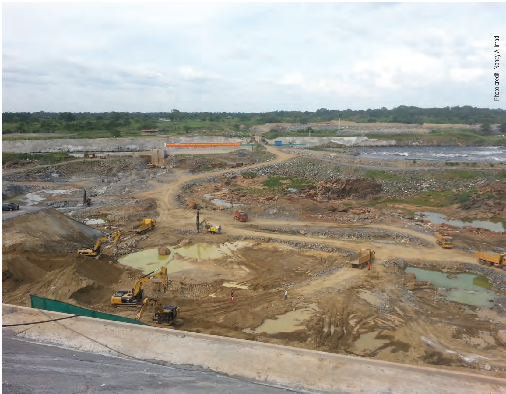
The 600MW Karuma Hydro Power Project under construction at Kyoga Nile, Karuma in Kiryandongo and Nwoya Districts
