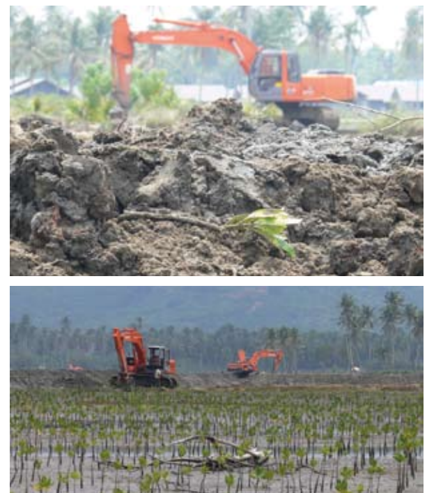
Figure 4.10. Construction of ditches (pond rehabilitation) has damaged the mangrove already planted (Lham Ujong village, Aceh Besar)
