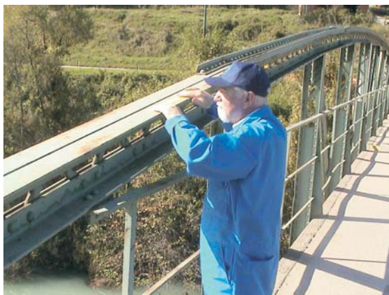
Special surface contamination studies were undertaken at 16 locations both near and on the bridge
