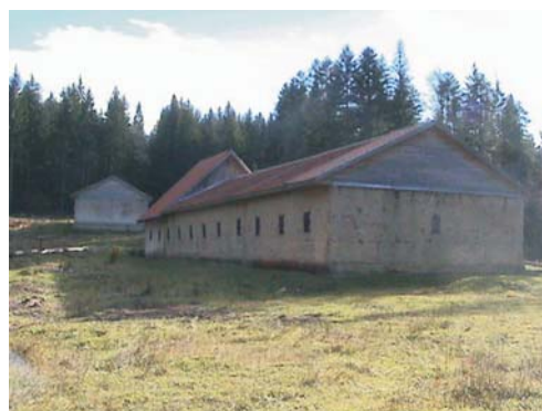
The repaired storage facilities are in a secluded area of the site
