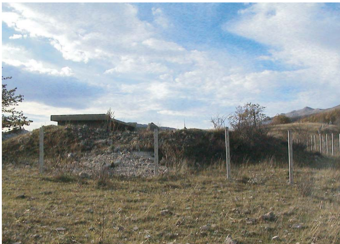
The destroyed water reservoir was most likely mistaken for a bunker
