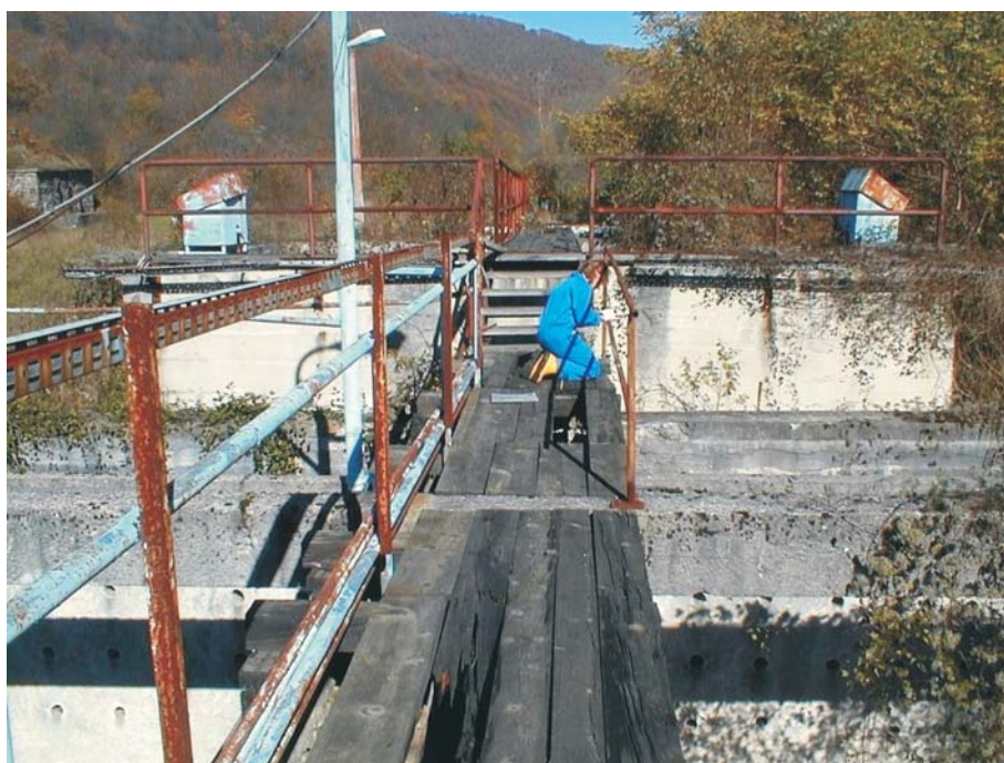
Water collected from the former water treatment plant showed no indication of DU
