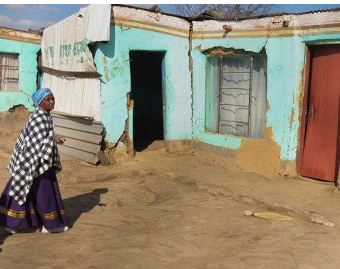
A home damaged by blasting from a mine operation 349
