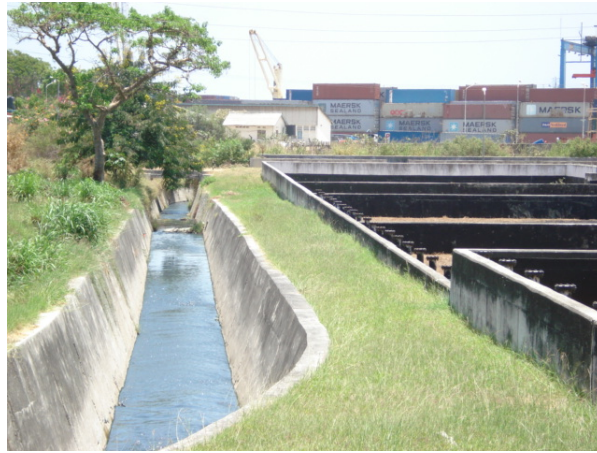
Figure 3.10 Wastewater from the Kipevu treatment plant in Mombasa draining directly into the Indian Ocean.
