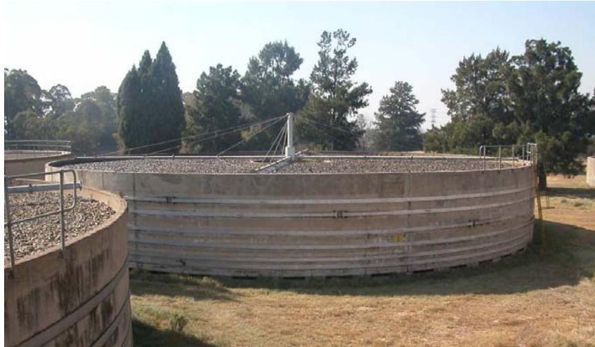
Figure 5: 6 Typical Trickling filter in South Africa
