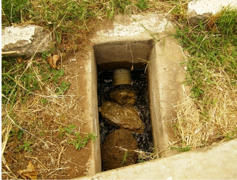
Figure 5: 4 Stone packed in the sewer inspection chamber
