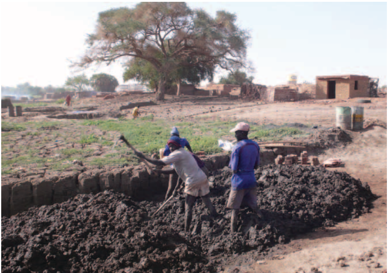
Most brick making in Sudan continues in the traditional, labour intense and energy inefficient manner. Resistance to change will stem mainly from a financial perspective for those controlling the brick making sector.
