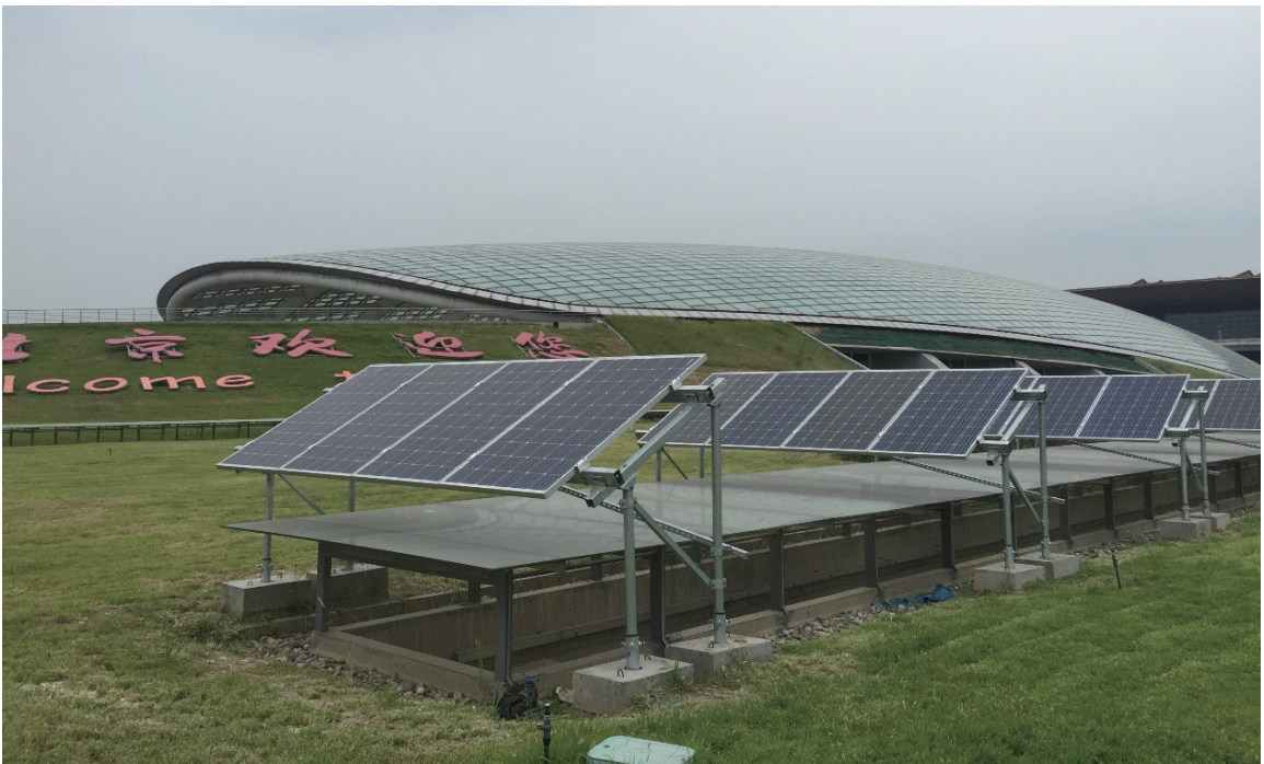
Fig. 4.7 Solar power project at ground transport center
