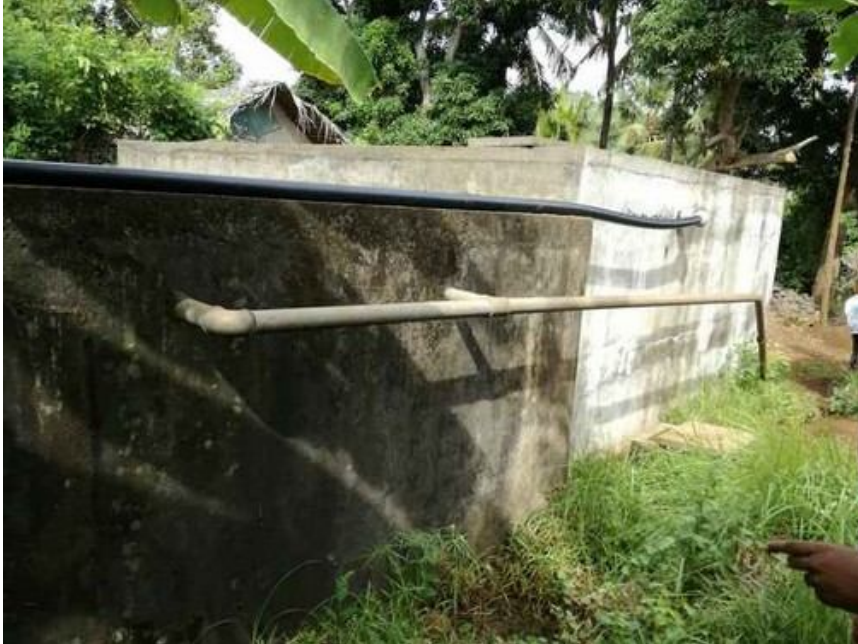
Lingoni-Mbatsé water supply scheme. New (right) and old (left) water reservoir. As the new reservoir has few connections, it overflows into the old reservoir (black, upper pipeline) making more water available for the existing distribution system.
