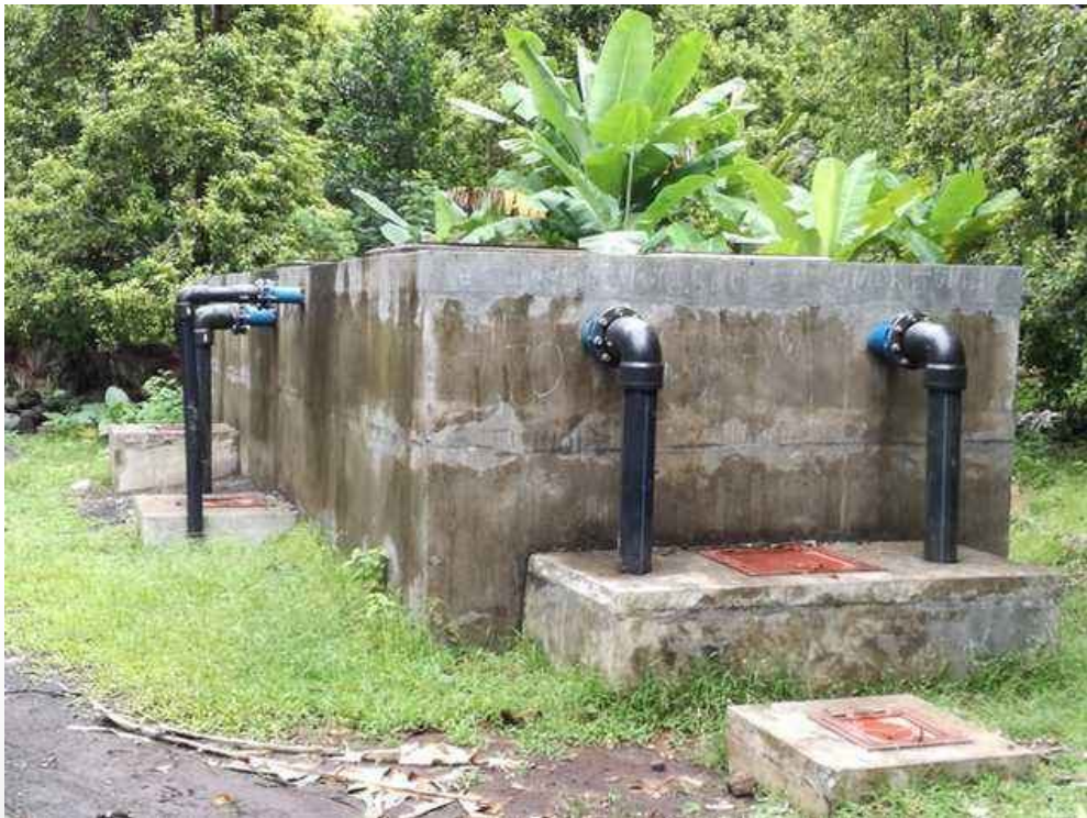
Filter Tank, Pomoni-Lingoni water supply scheme
