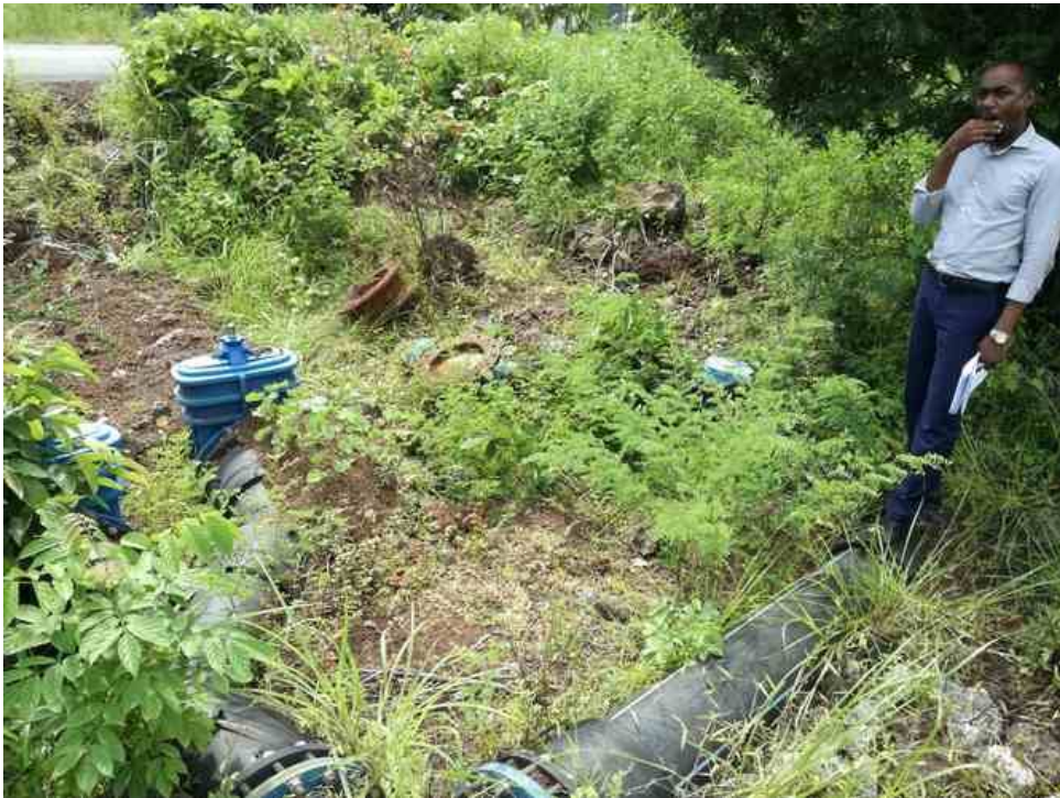
Airing valve, Moroni water supply project.
