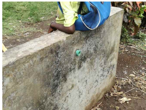
Broken school stand-post, Pomoni
