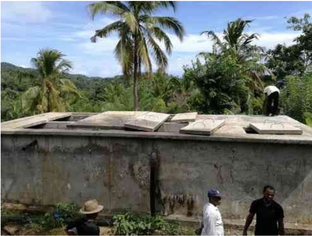
Slow Filter, Lingoni-Hoani water supply scheme. The covers turned out to be too heavy to manage. The plan is to substitute them with lighter covers.
