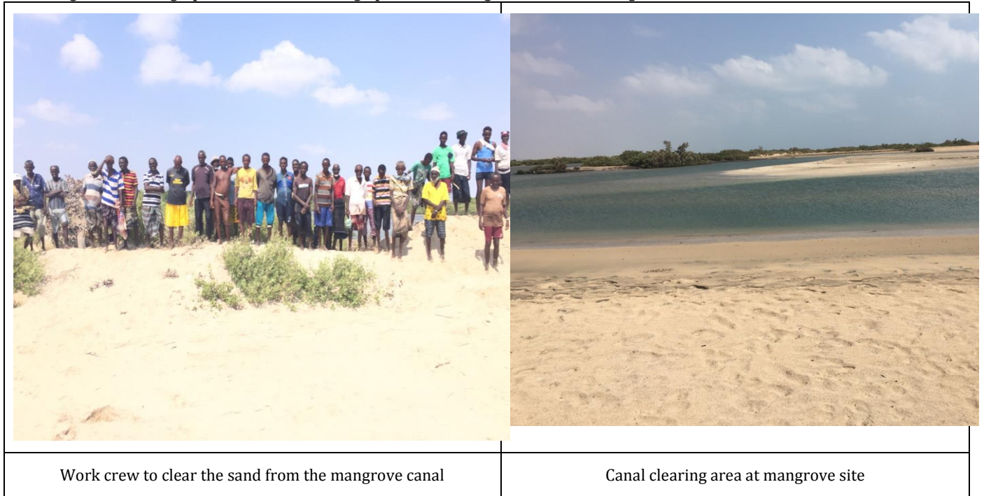
Figure 13: Photographs at the Canal Clearing Operation at Mangrove Site in Khor Angar
