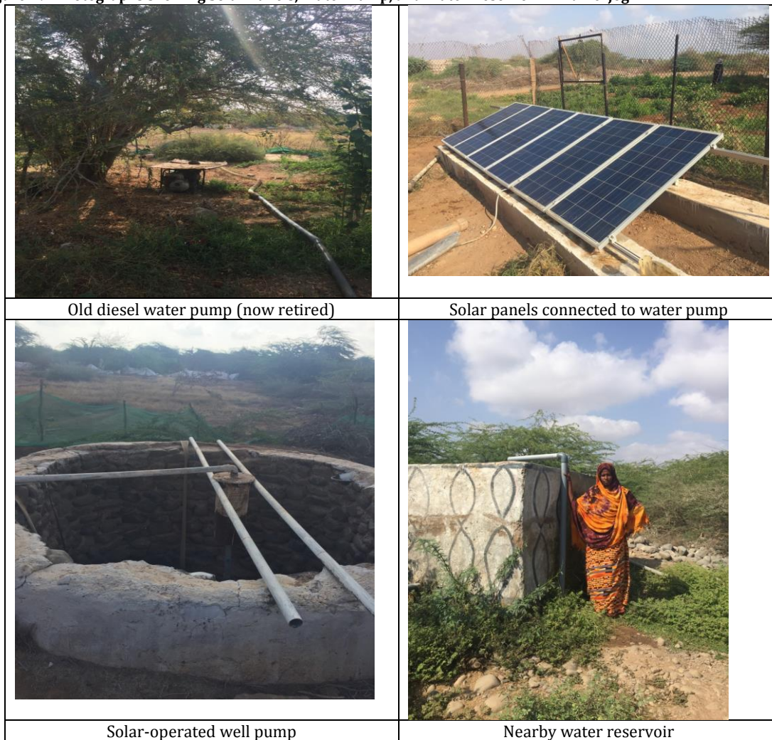
Figure 19: Photographs showing Solar Panels, Water Pump, and Water Reservoir in Damerjog
