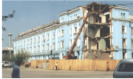
Figure 1. Destruction of the building in the centre of Yakutsk (Eastern Siberia), 1999.
