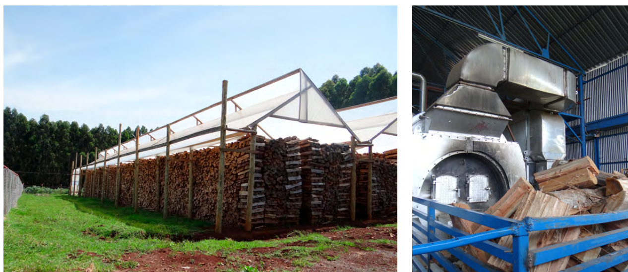
FIGURE 19: Wood drying before use in a boiler fed by woody biomass at Finlays estate (Kericho)
