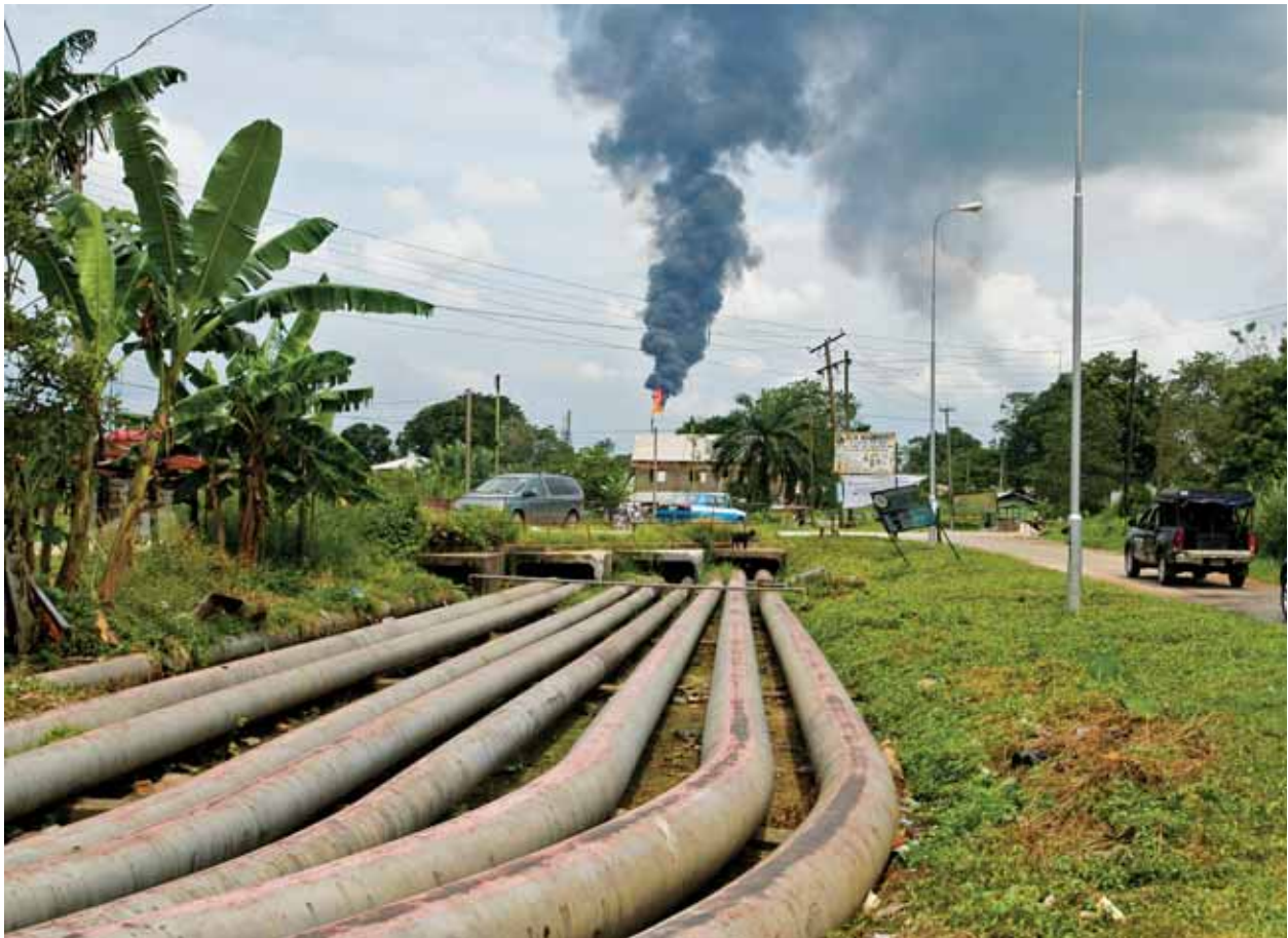
Pipelines in neighbouring Okirika LGA. The environmental impacts of oil operations are a shared legacy
