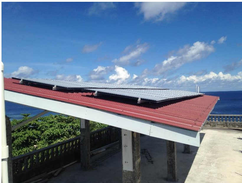
Figure 7 5kW solar installation at the at the roof of the Od'n Aiwo Hotel in Nauru
