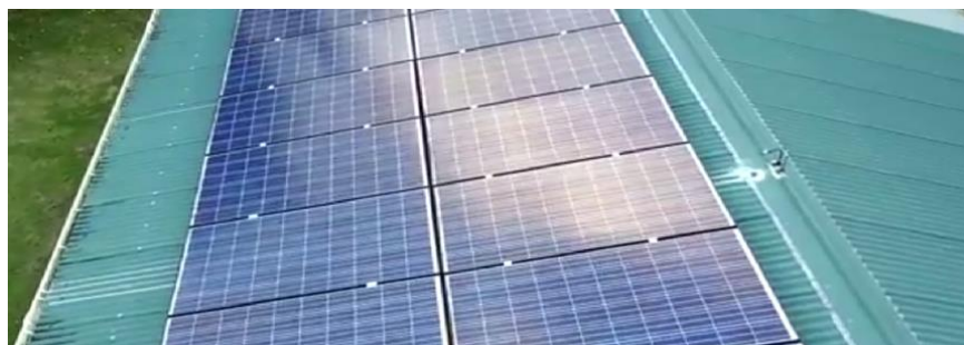
Figure 8 5kW solar installation at Stone Villa in Alofi, Niue
