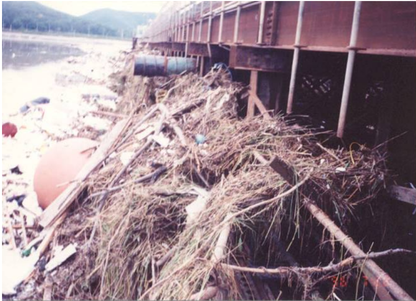
Figure 9. Marine litter at the 2 nd Gangwha Bridge, Incheon City (1997).
