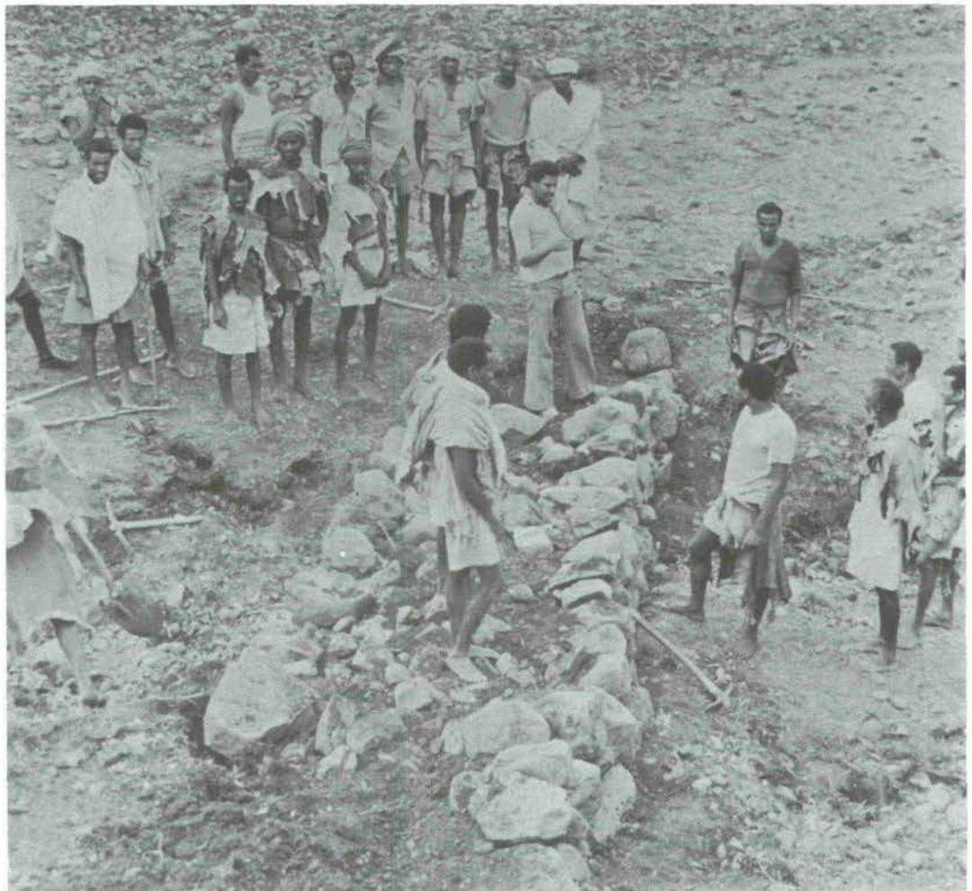
WFP has been funding a very successful programme of terracing in Ethiopia. Here a technician explains to the workers how to build the foundation for a terrace. (UNEP/Charles Stewart)
