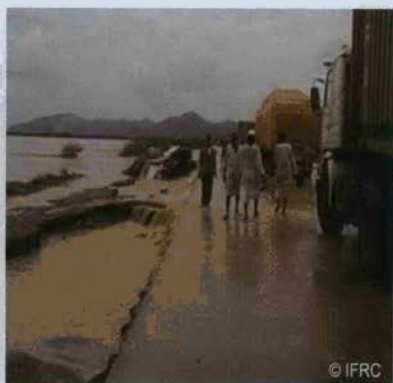
Flood damage in Sudan.
