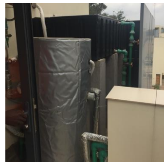
Solar water heater tank (collector plate on roof) with insulated pipes
