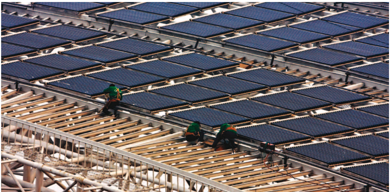
Solar collectors on the rooftop of a company headquarters, China
