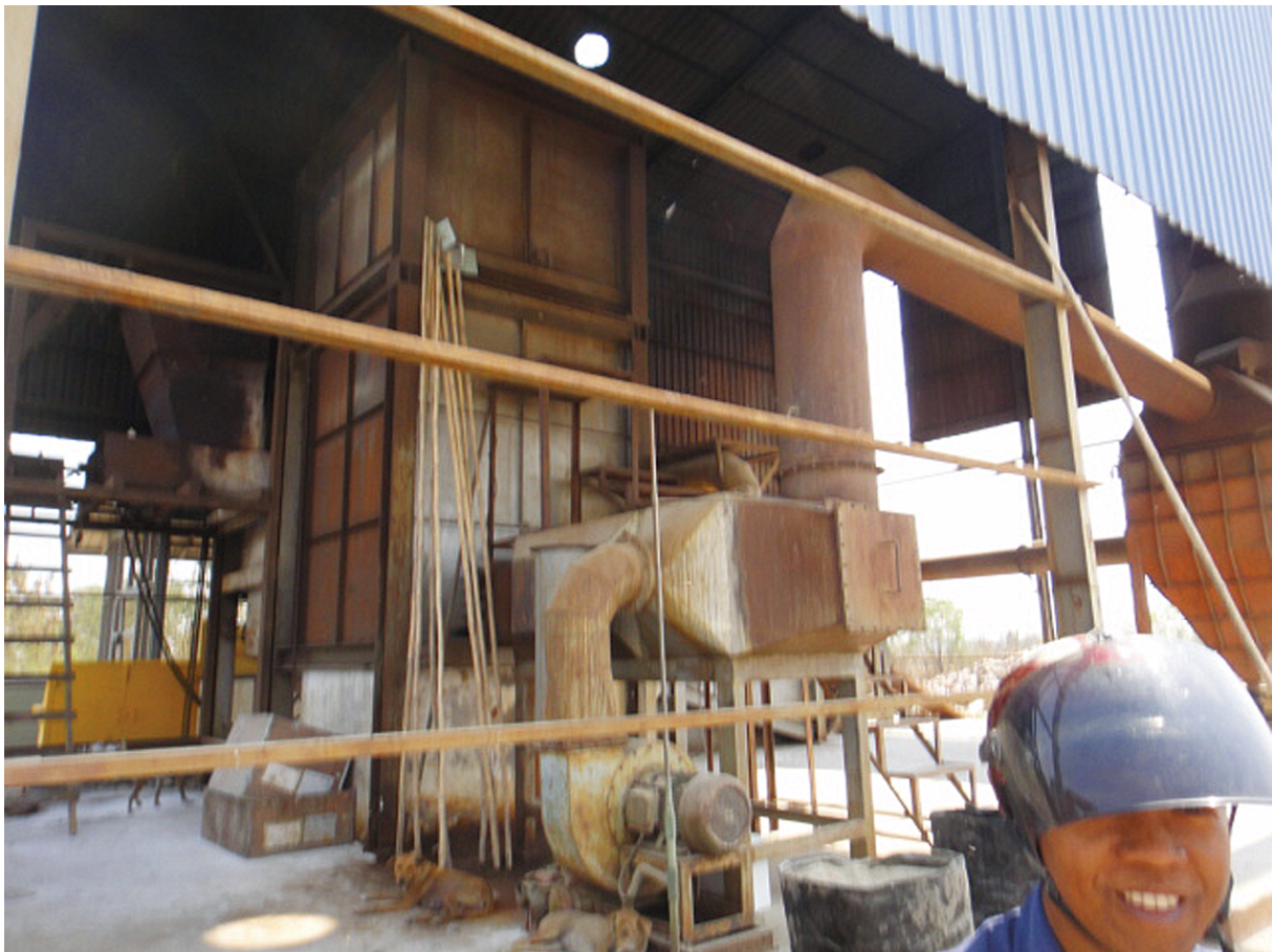
Figure 11: Incinerator stopped in operation. Source: IGES, 2016
