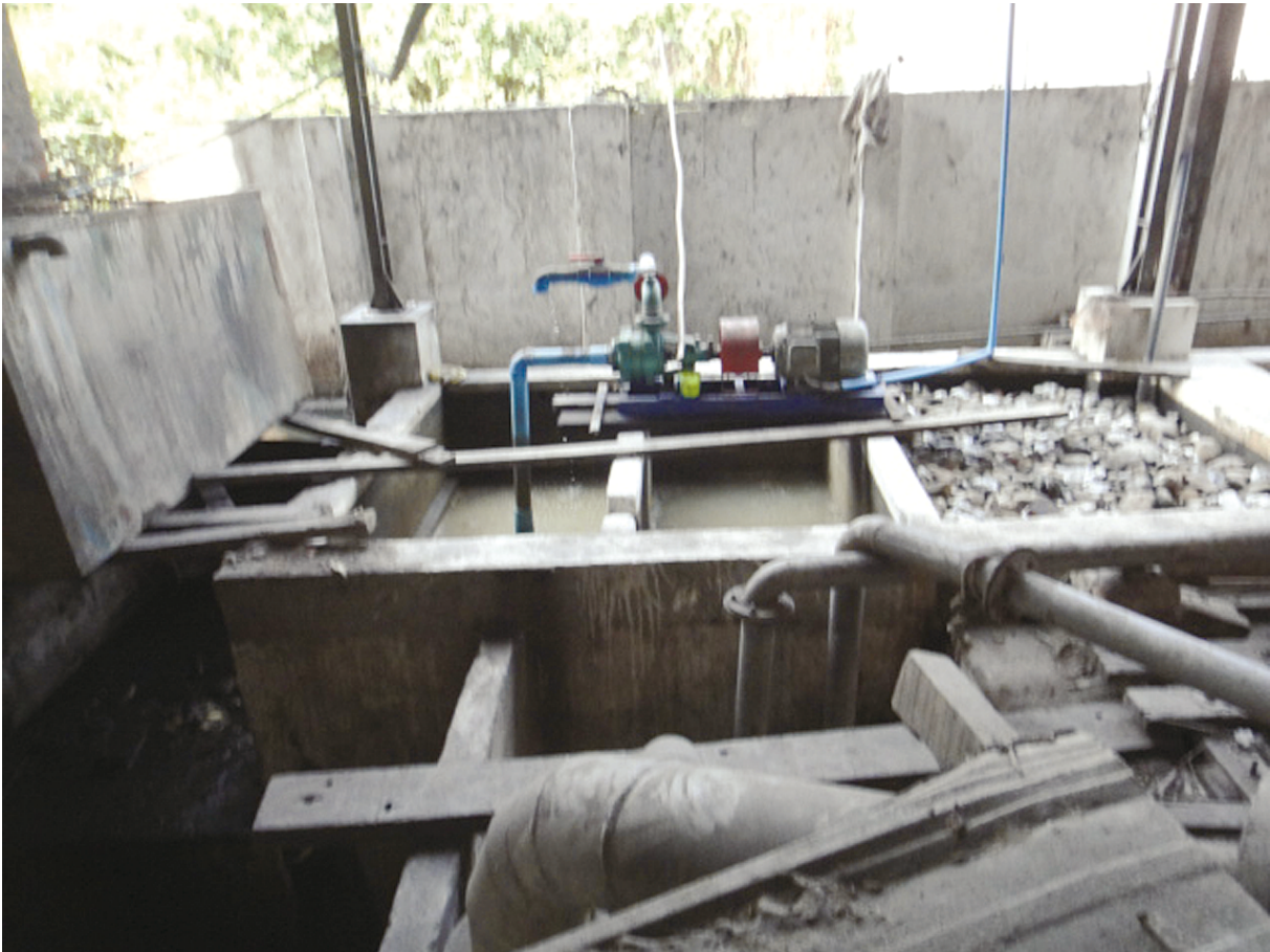
Figure 6: Waste water treatment plant in a factory. Source: IGES, 2016
