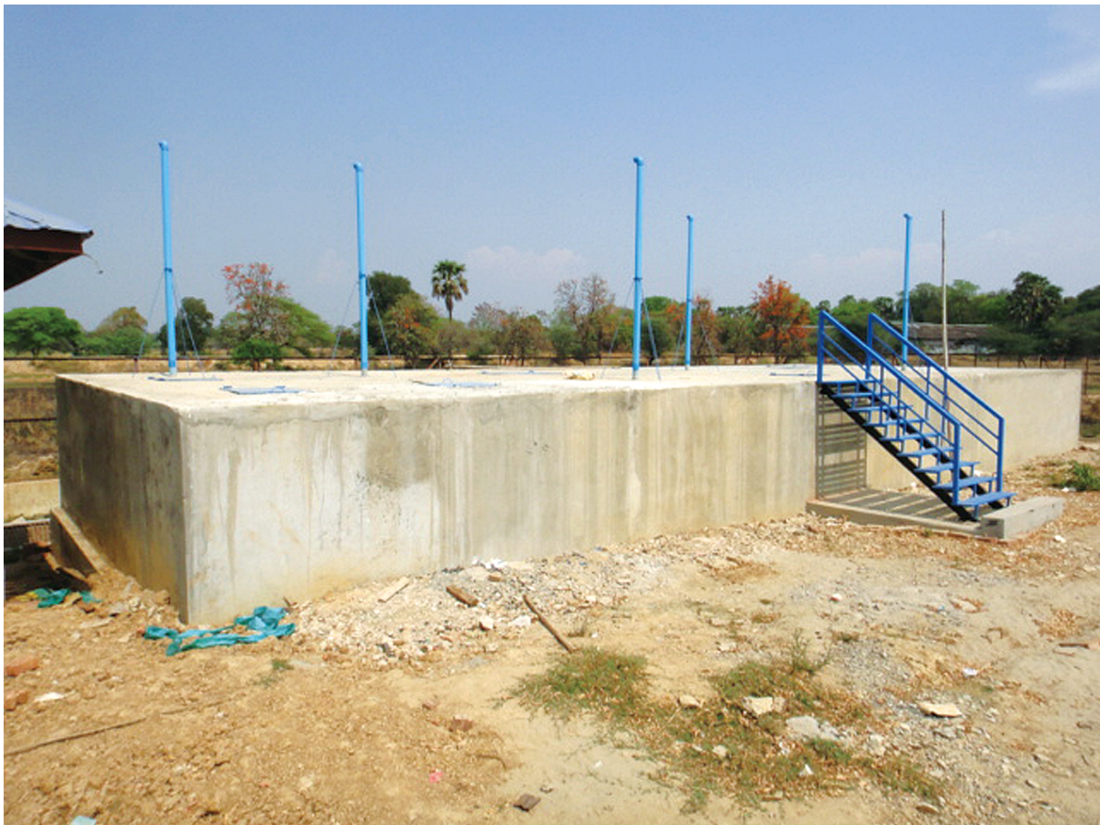
Figure 12: Newly built waste water treatment plant in Mandalay. Source: IGES, 2016
