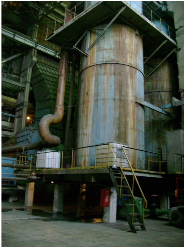
Figure 1. Wet PM scrubber.
