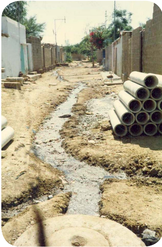
Orangi Pilot Project Research and Training Institute (OPP-RTI)
