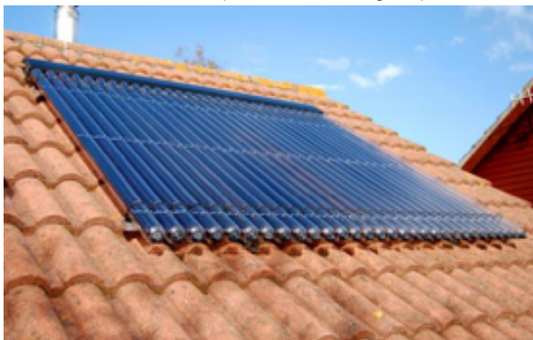
FIGURE 9 • ROOFTOP SOLAR WATER HEATERS/SOLAR THERMAL COLLECTORS ( YouGen United Kingdom )
