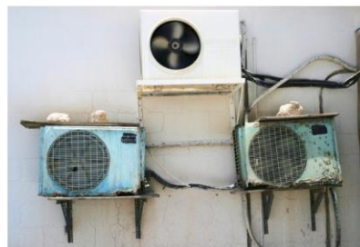
CFCs from older cooling units are not covered by the Montreal Protocol. Credit: Jason Larkin/Construction Photography/Aviation/Getty
