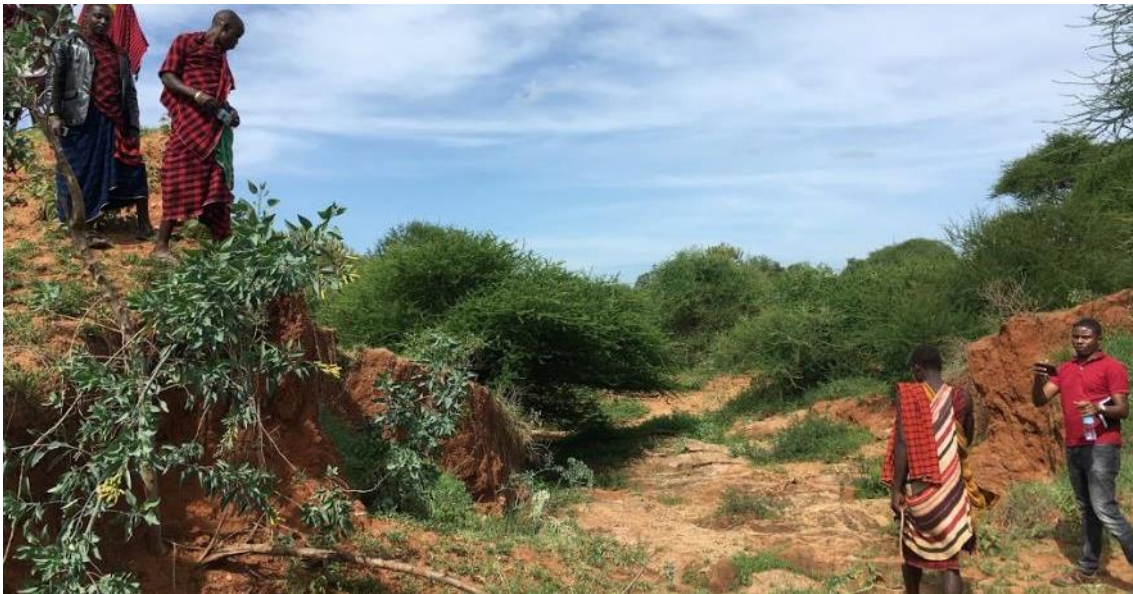
Figure 47: Breached wall observed at one charco dam
