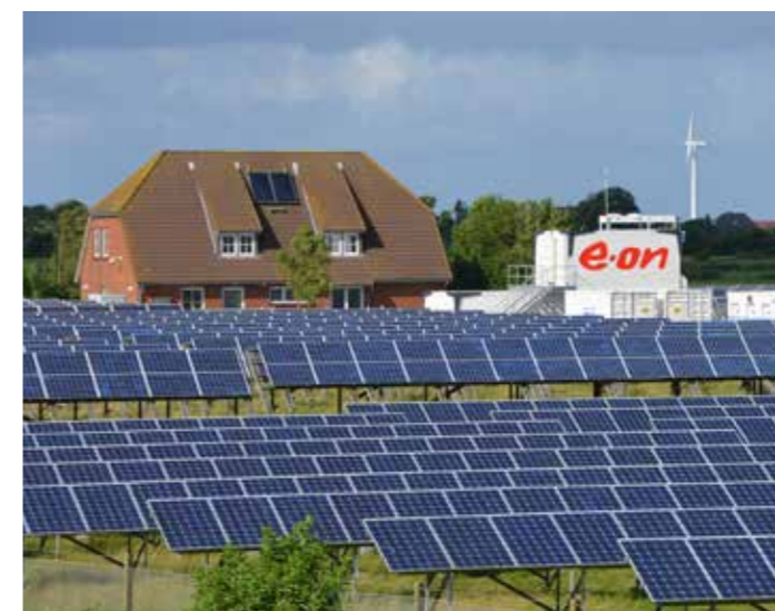
PV and Battery storage system at Pellworm Island (Photo: E.ON)
