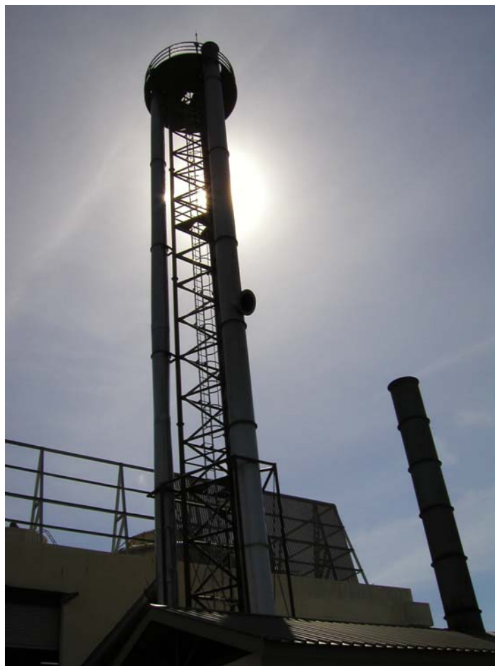
Picture 2. The chimneys of MWI at RIPAS hospital
