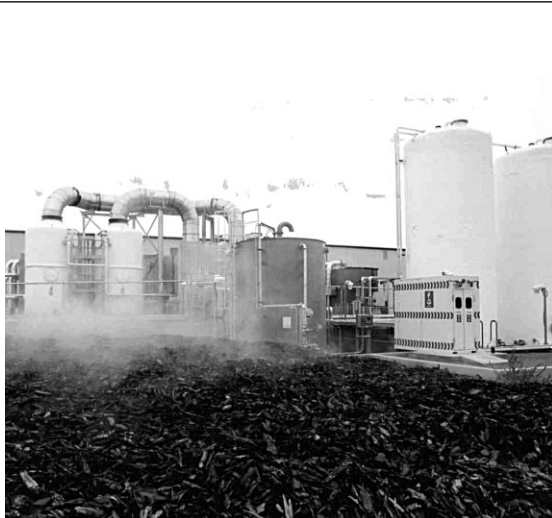
The Edmonton Co-Composting Facility Courtesy: Stantec
