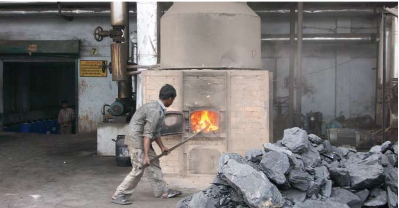
Coal boiler in India
