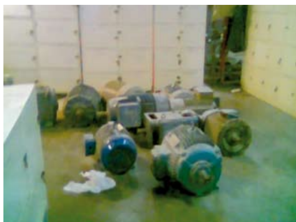
Before: Housekeeping lapse – poor storage of equipment
