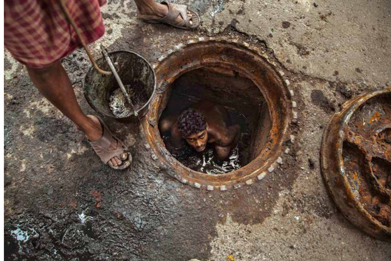
Figure 5. A sewer worker cleans the drainage system of the metropolitan city of Kolkata, India, without proper protective Equipment (Photo credit: Sujan Sarkar with courtesy of Photoshare).
