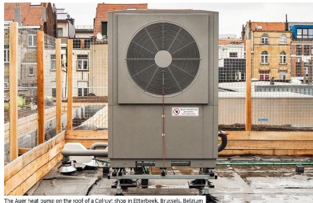
The Auer heat pump on the roof of a Colruyt shop in Etterbeek, Brussels, Belgium
