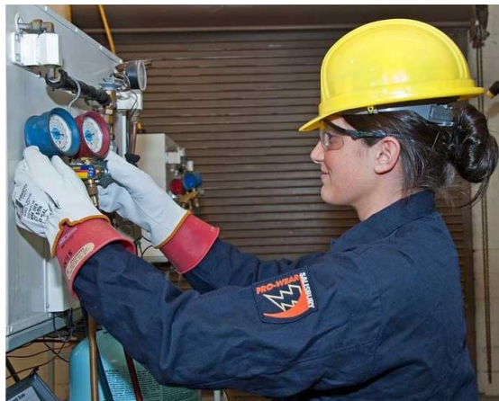
U.S. Air Force Senior Airman Stephanie Holt, 366th Training Squadron, HVAC/R Apprentice course, checks the HVAC system's refrigerant pressure at Sheppard Air Force Base, Texas. (Courtesy of Picryl)
