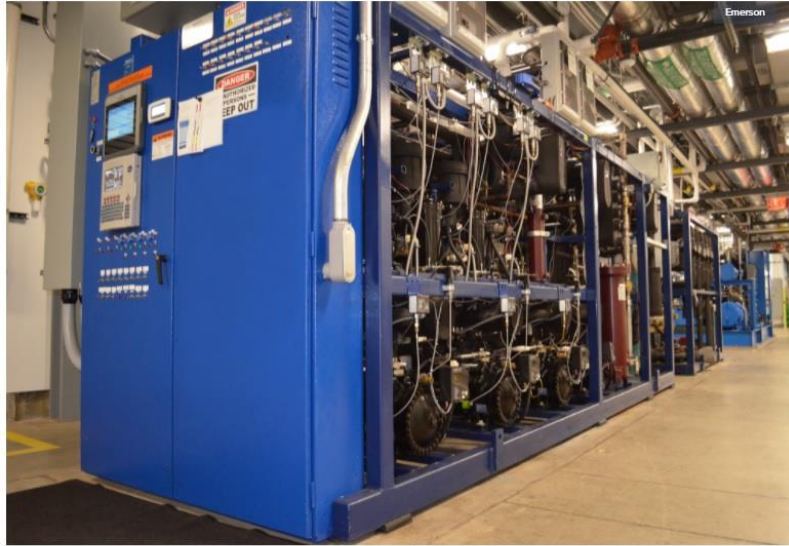
CO 2 transcritical booster systems are subject to declining efficiencies in warm ambient climates, but manufacturers have developed a variety of strategies to maintain efficiency levels.
