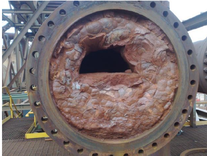
Figure 4: Example of solid waste accumulated on the inner surface of a mismanaged pipeline Image provided by Qa3.
