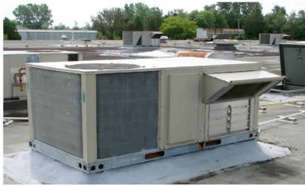
Roofing HVAC unit with view of fresh air intake vent. Credit: Wikimedia
