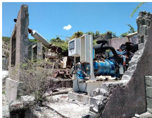
Figure 6: Port-a-Piment grid 230 kVA and 250 kVA gensets
