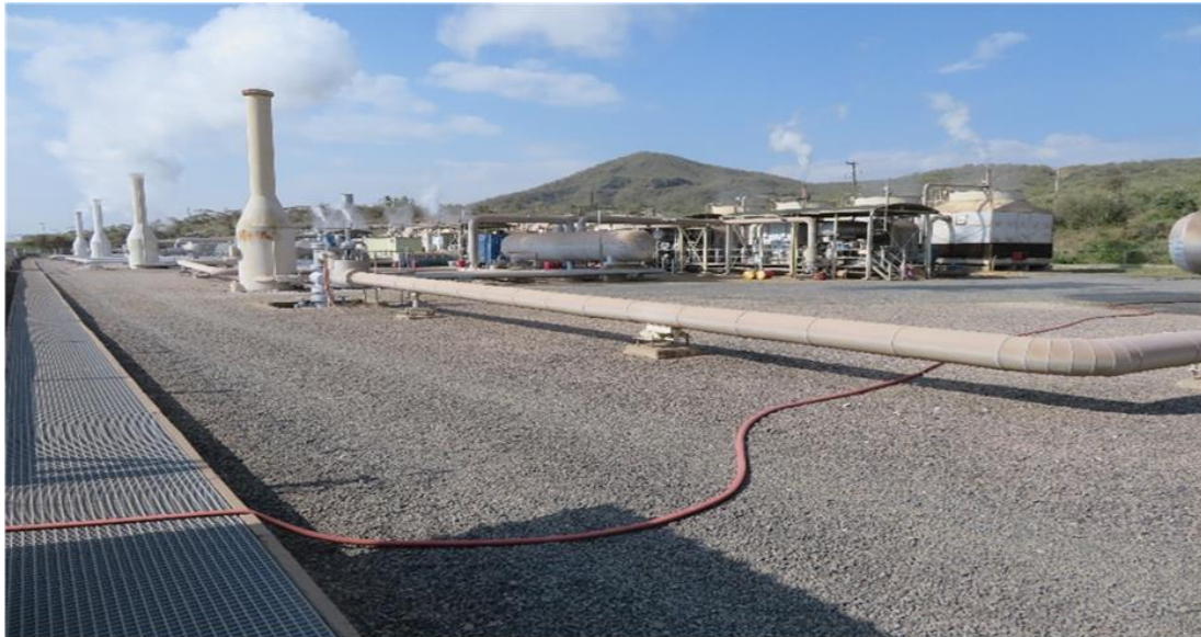
Photo: Geothermal Power Plant's few 6 MWel at KenGen in Kenya (Source: Runar Magnusson, 2016)
