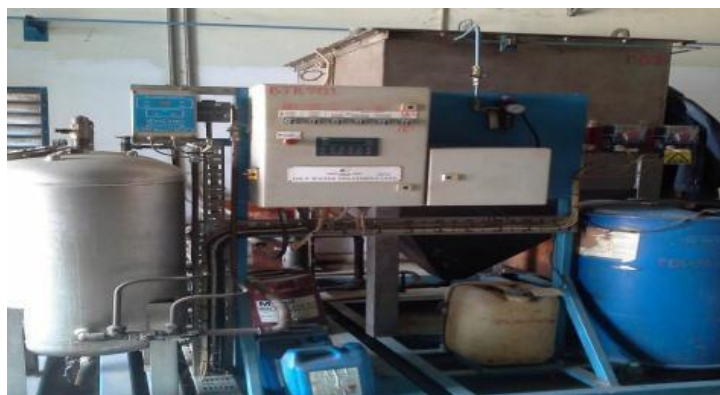
Figure 12: Advance oily water treatment unit being used in electric power generation in PPM
