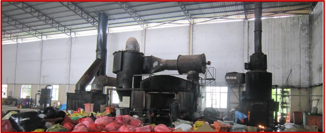
Figure 12 : Type of modern incinerator for healthcare waste in Phnom Penh
