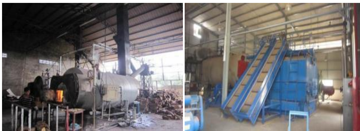
Figure 17: Overview of one of clean wood fired power boiler being used in Cambodia industry
