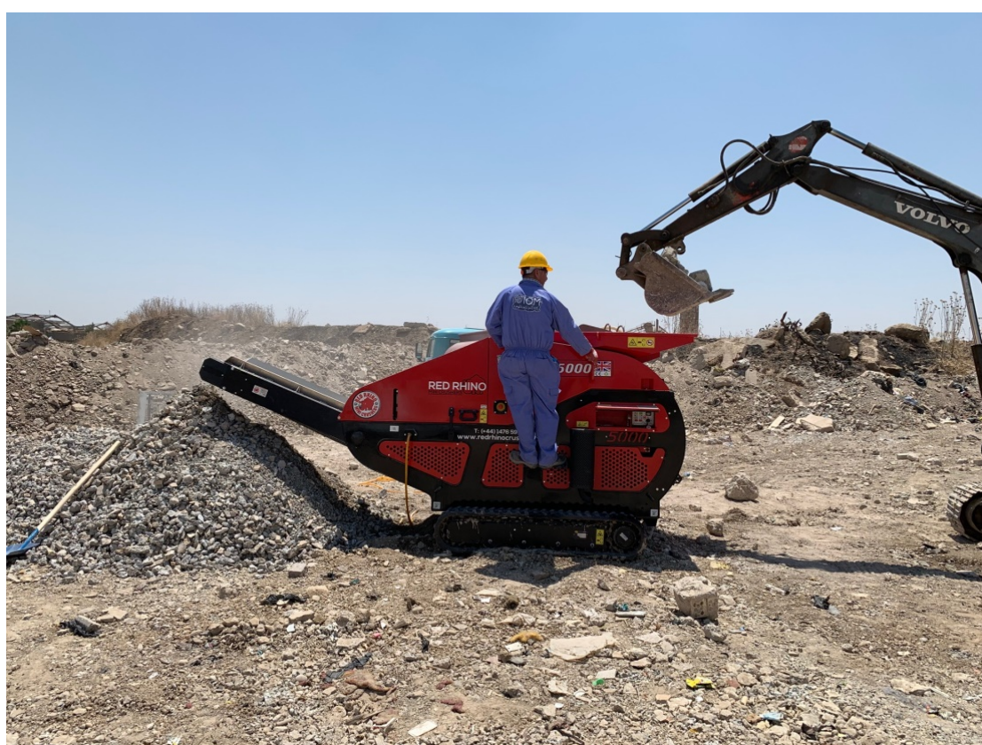
Figure 1: Small scale crushing of debris by the International Organization for Migration (IOM) at the Mazen Debris Recycling Pilot Site in Mosul
