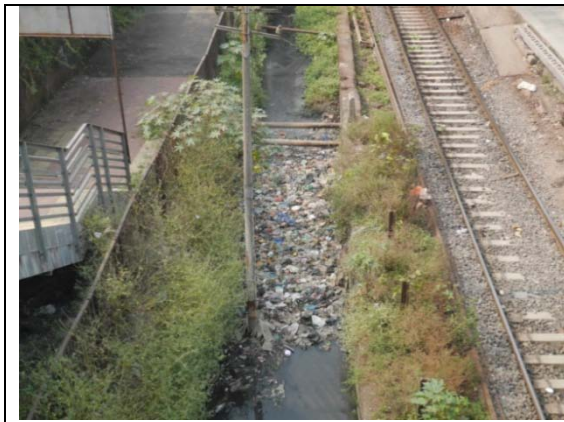
At Govandi Station (19° 03' 17" N and 72° 54' 56")- Plastic Clogged into Small Drain
