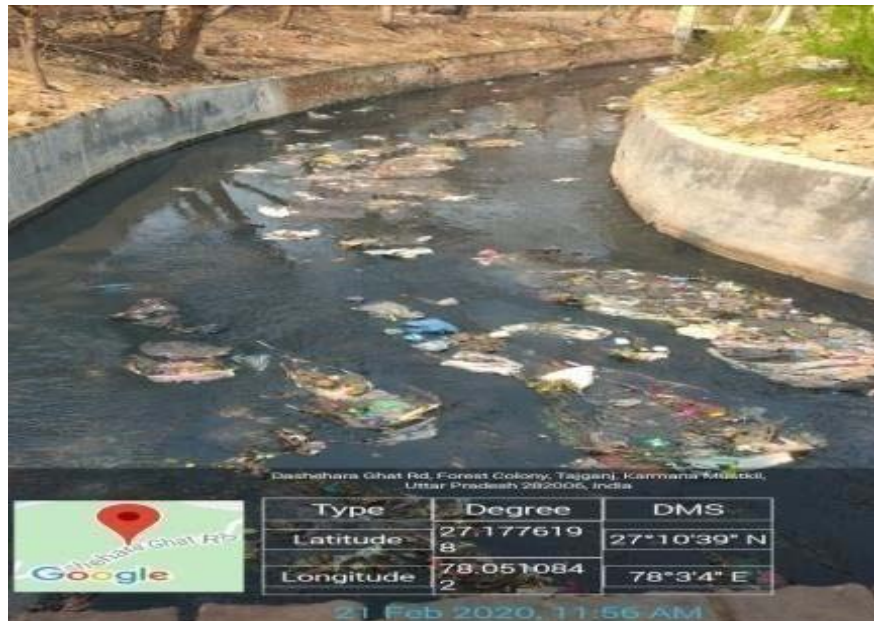
Figure A1.46: Mixed Wastes is Floating in Open Drain
