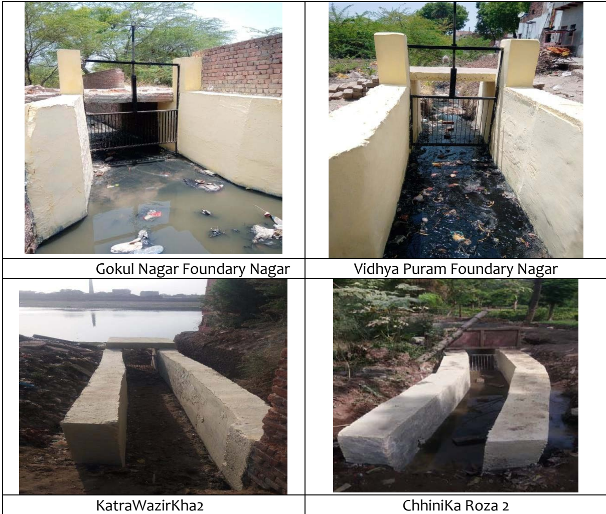
FigureA1.50: Drain Barrier in Agra
