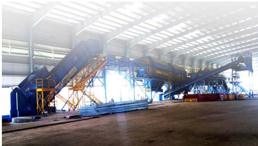
Photo Plate No.4.26 Material Recovery Facility (MRF) at Kanjur Processing Plant.
