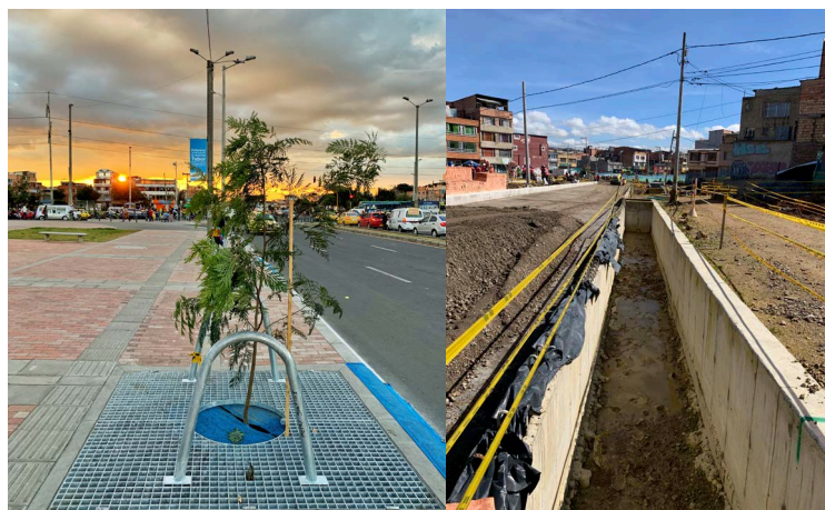
Figure 5.4: Floodable pits on Rincon Avenue, Suba, Bogota (left) and infiltration ditches with bioretention zones under construction on Rincon-Boyaca Avenue (right).
