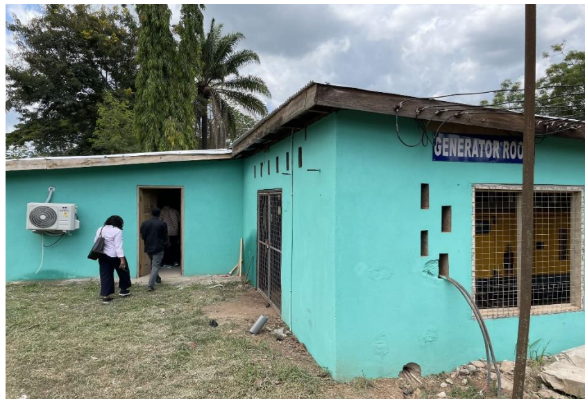
Figure 12: Photo from diesel emergency electricity generation station at St. Marys Hospital in Ghana (Photo: Yamini Jain, May 2023)
