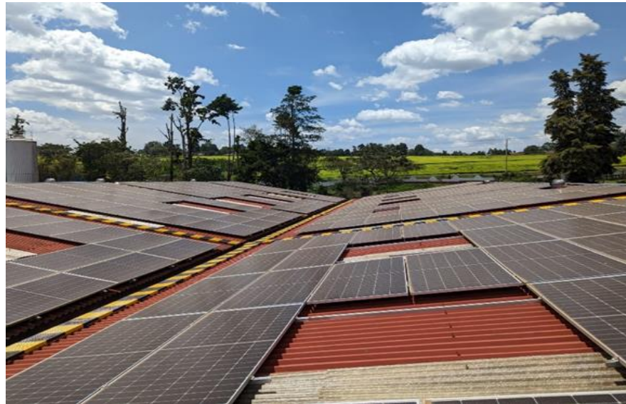
Figure 1: Solar PV installations on the roof of SOTIC company in Kenya (Photo: Carolina Merighi, January 2023)
