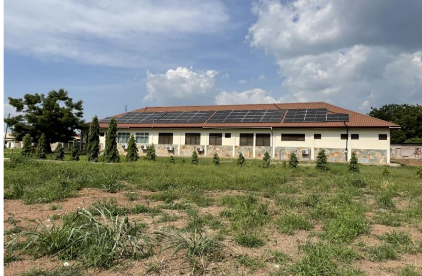
Figure 6: Photo from Holy Family Hospital with its PV installations in Ghana (Photo: Yamini Jain, May 2023)
