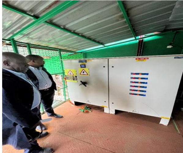
Figure 7: Solar PV installations at Fresha Dairy Farmers Co-operative in Kenya (Photo: Carolina Merighi, January 2023)
