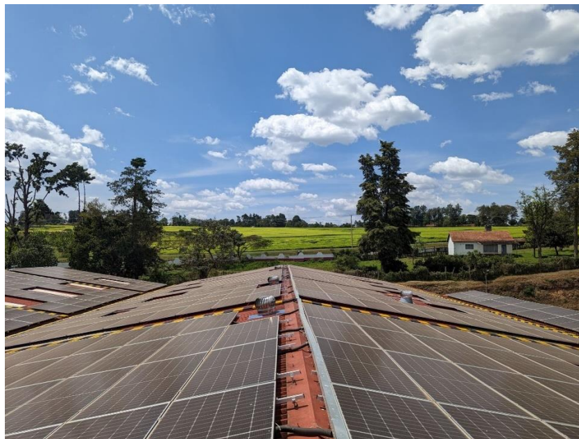
Figure 16: Photo from photovoltaic installations at NKCC, New Sotik Market in Kenya (Photo: Yamini Jain, January 2023)
