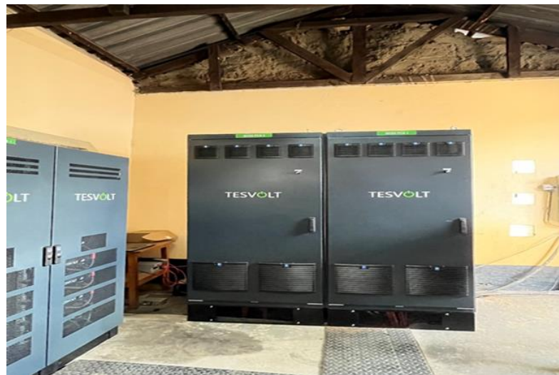
Figure 15: Solar PV installations (converter from DC to AC) at Fresha Dairy Farmers Co-operative in Kenya (Photo: Carolina Merighi, January 2023)
