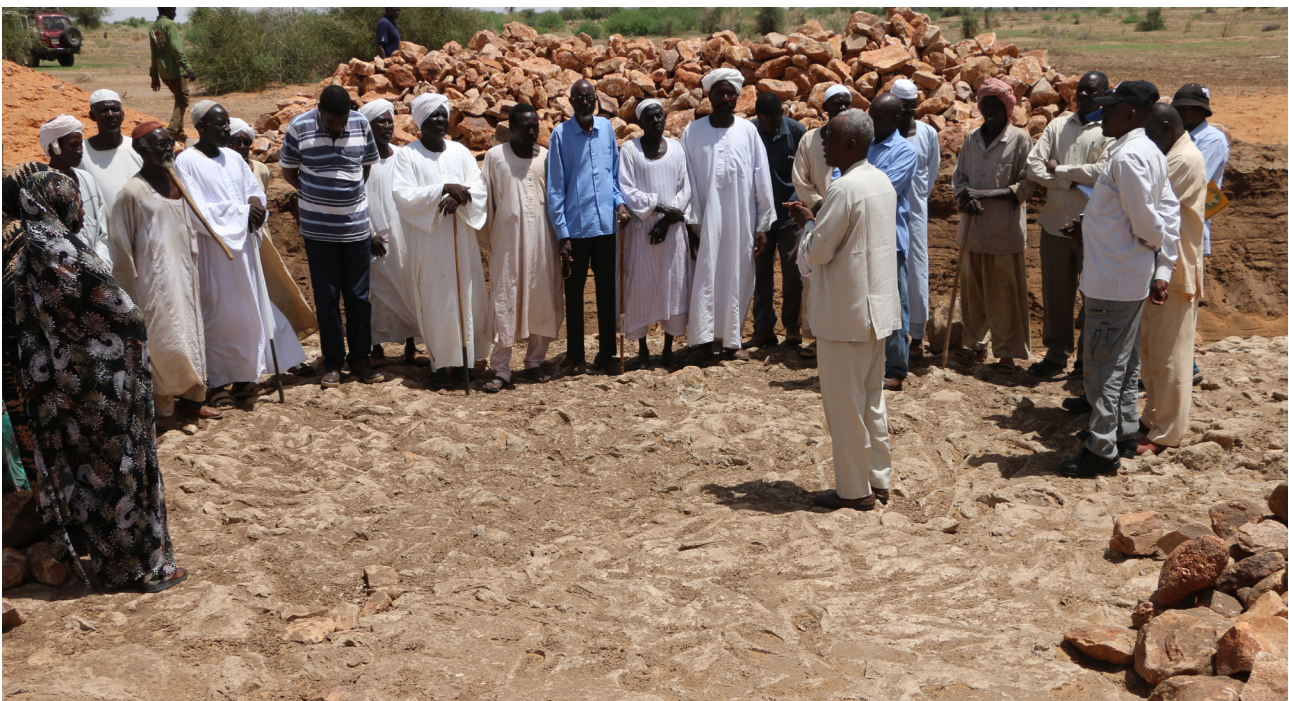
Involving communities in all stages of weir construction fosters a sense of ownership and ensures the sustainability of the project's interventions. Photo credit ©Practical Action
