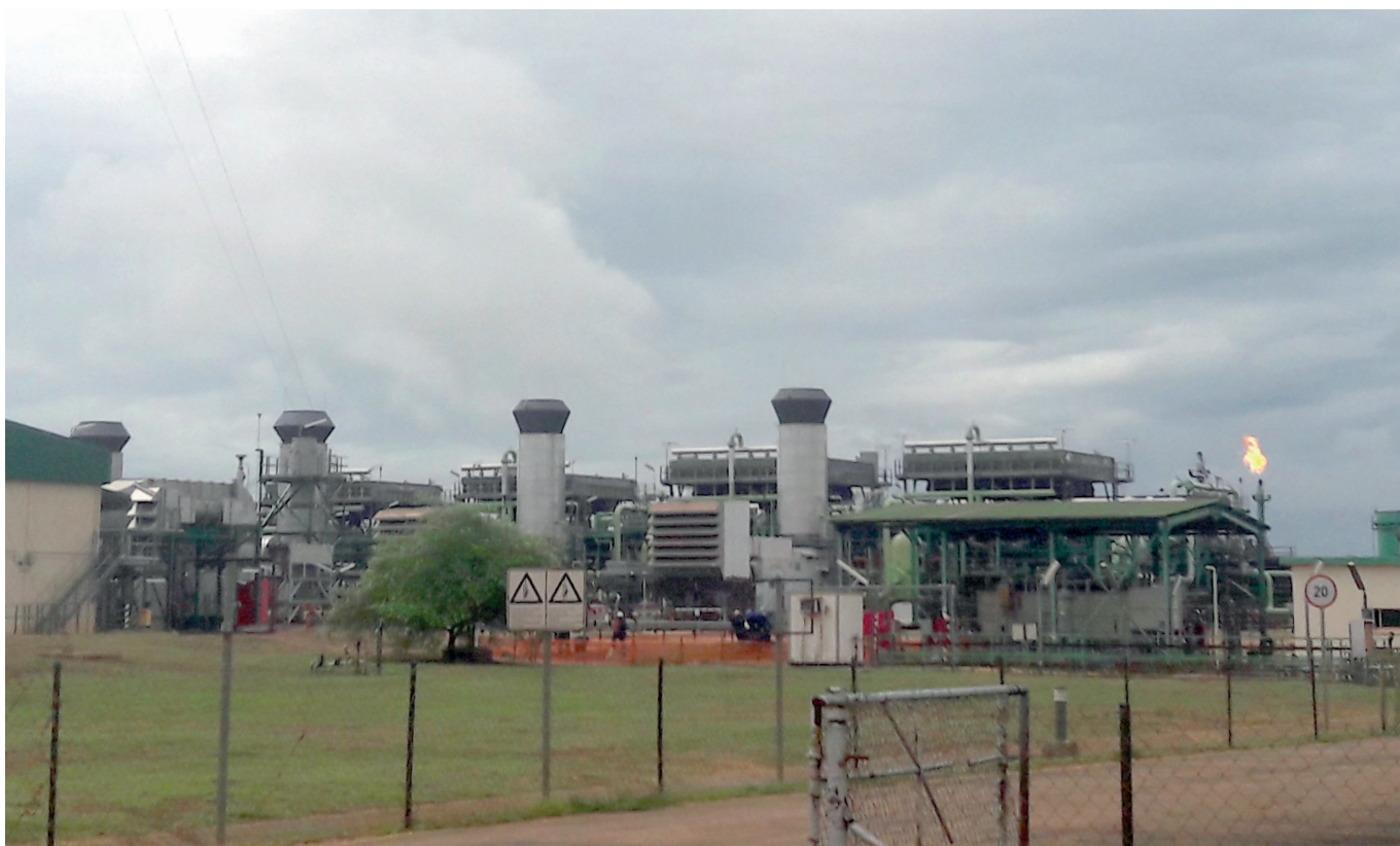
FIGURE 2. Sasol's Central Processing Facility close to Vilanculos, in operation since 2004.
