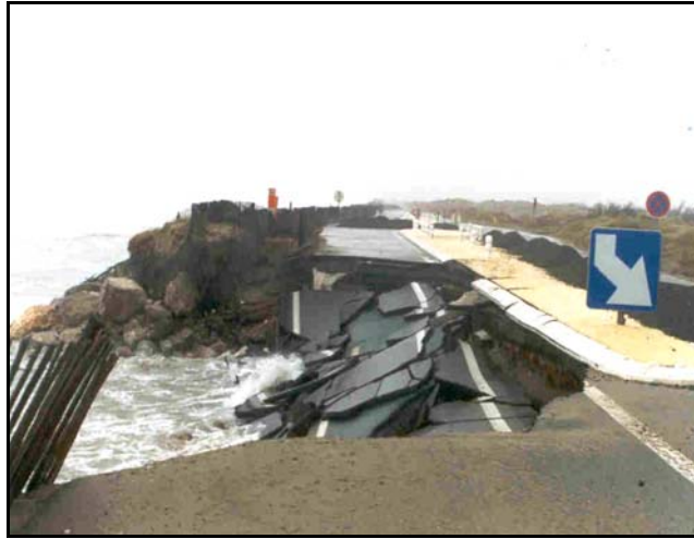
Figure 5. The impact of extreme meteorological events (storms, sea surges ...) on roads and structures on the Mediterranean coastline
