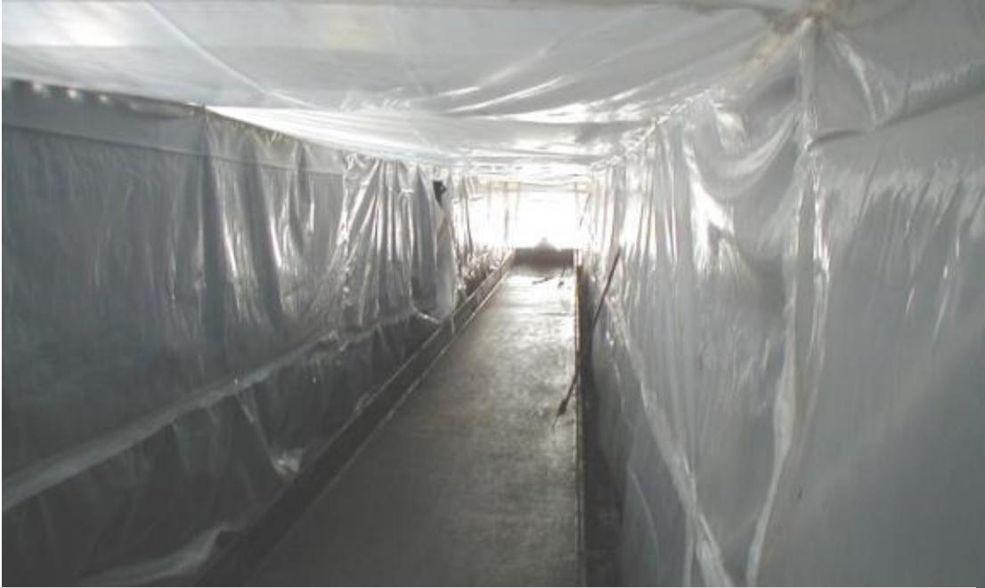
Cell confinement (connected to the air treatment unit)
