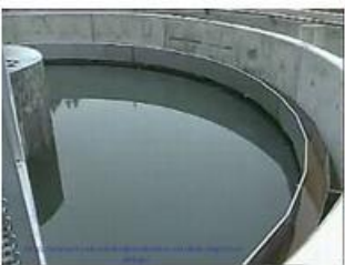
Waste water treatment plants
