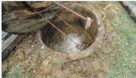
Location potentially contaminated with PCBs, Elektrodistribucija Zenica TS 35/(20)10 Jelah
