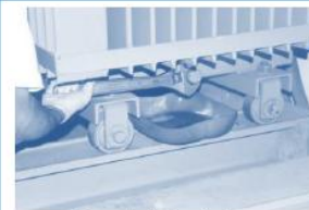
Open drain tap/valve (usually by local electrical technician)
