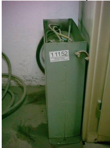
Picture 56: Inventoried and labelled capacitor
