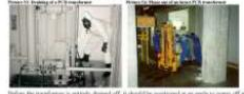
Photo 11: Phase out of transformer (transformer Phase out) (Photo 11: Phase out of transformer)
