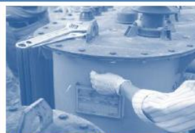
Affix sampling label on transformer (after cleaning the surface)
