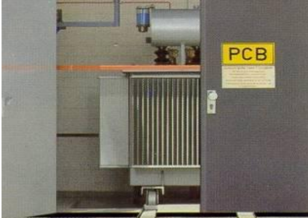
Picture 38: Labelling of a transformer room door
