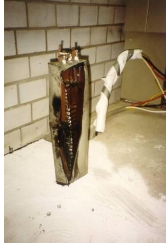
Picture 50: Burst capacitor
