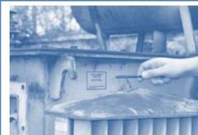
When test results are available, re-label the tested transformer
