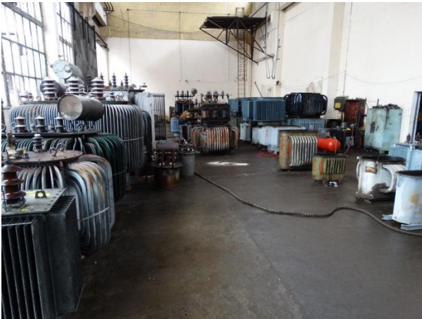
Picture 40: Transformer maintenance area
