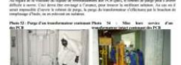
Photo 12: Phase out of transformer (transformer Phase out) (Photo 12: Phase out of transformer)
