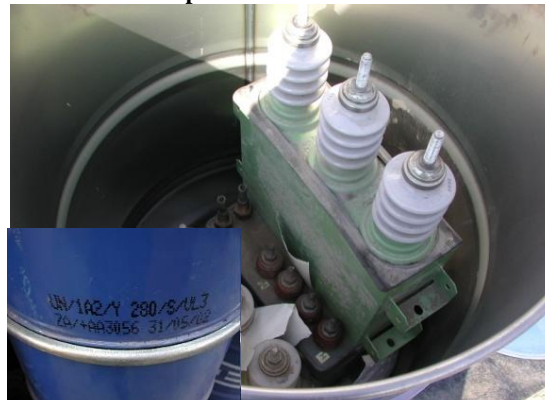
Picture 68: PCB capacitors in steel drum
