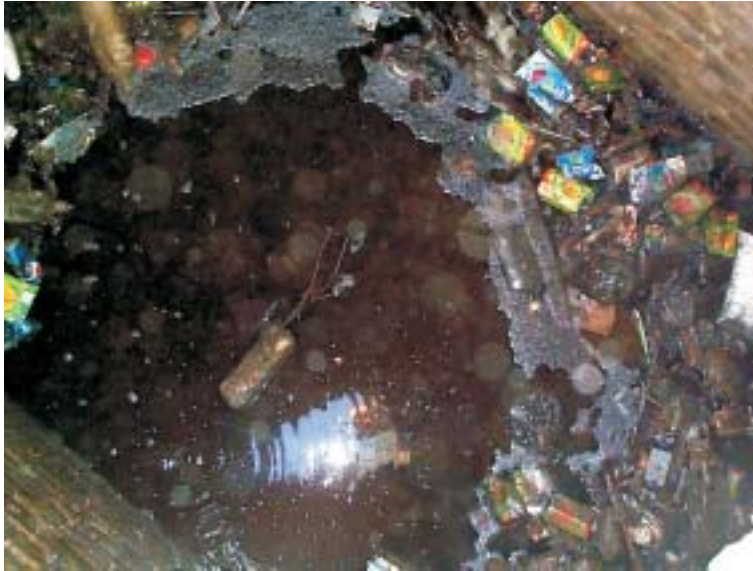
Well in Mazar-e-Sharif Civil Hospital filled with medical wastes.
